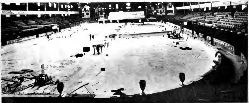
FIG. 30. ON JUNE 11 THE TIE WAS POSITIONED. THE FINISHING WORK ON THE POOL WAS BEING COMPLETED. THE ELECTRIC WORK WAS BEING PUT IN PLACE. THE WATER MAINS WERE BEING LAYED IN PLACE. THE CONCRETE WAS BEING SET.
